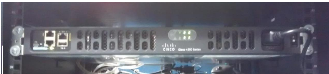
Figura 16: Router Cisco 4500 series parte 1
