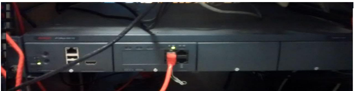
Figura 17: Router Cisco 4500 series parte 2
