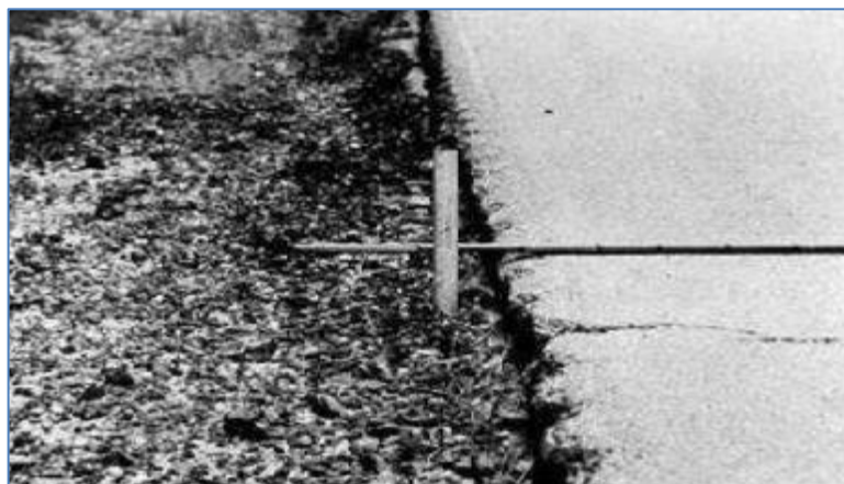
Figura 100. Desnivel carril – berma – alta severidad
