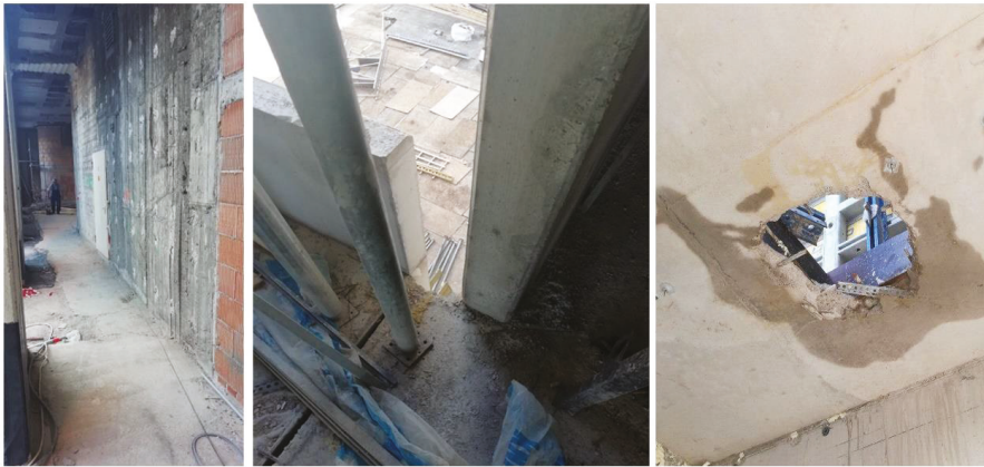
Figure 12. Case study, shots of the failed inspection lots: wall concrete surface with honeycombing (left), wall cross-sectional geometry (center), hole in a slab (right).
