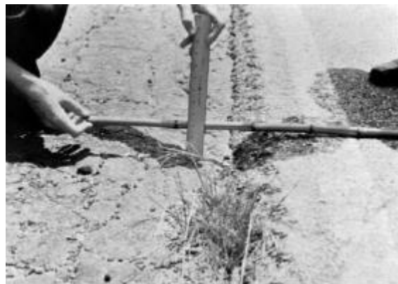
Figura 30: Desnivel carril/berma - severidad media
