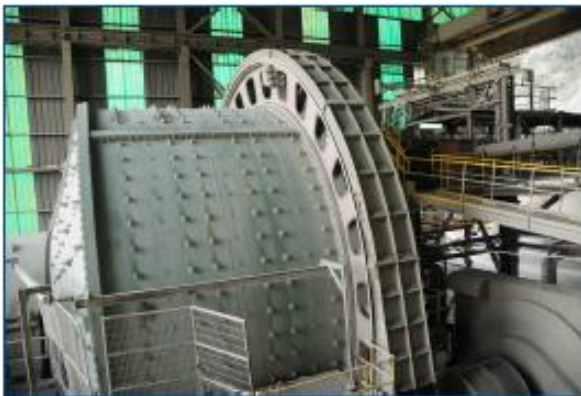
SAG and Ball mills at an ore processing facility – typically the mill drives, the mill gearbox and mill bearings are monitored. Loss of one SAG mill could result in a significant production shortfall.
