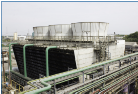
Cooling Tower Fans – typically the fan motor and gearbox are candidates for monitoring. Loss of a cooling tower fan gearbox could limit available cooling and reduce production capacity.
