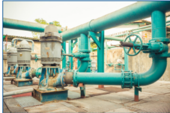
Vertical Water Pumps – pump drive and pump bearings are the components monitored. Loss of one pump could affect the ability to meet peak water demands.
