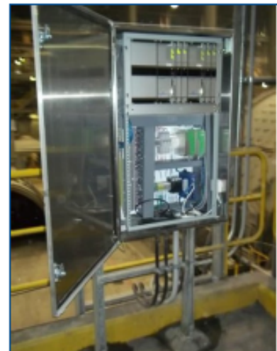
A 48-channel AMS 6500 deployed in a A6500PRE-SS-WM-IC wall mount enclosure, monitoring SAG and Ball mills at an ore processing facility.
