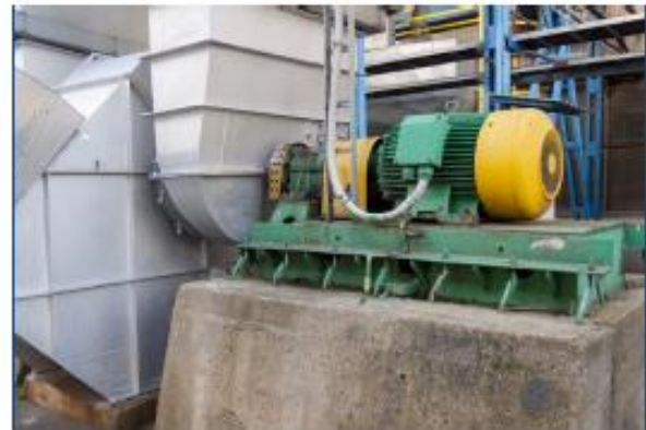
Large Centrifugal Fan – typically the fan drive and fan bearings are the components monitored. This fan does not have a backup.
